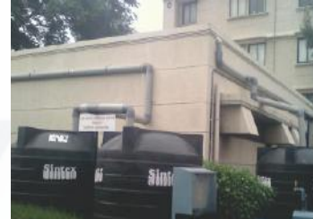
Rain Water Harvesting
